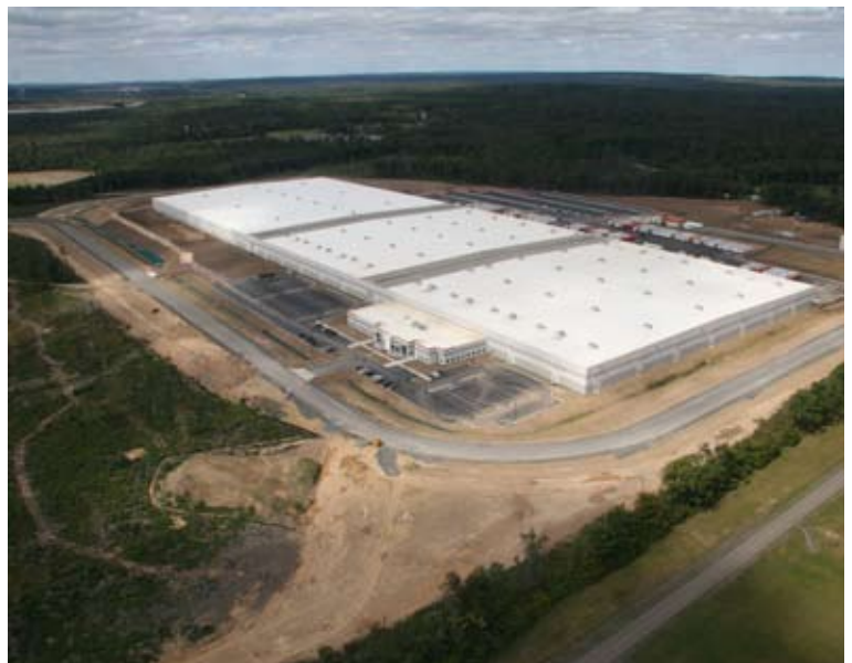
An aerial photo of the new Johnson & Johnson distribution center taken in late 2007. An artists rendering depicting the center's expected appearance upon completion is shown above.
